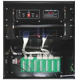
SME-144D (Telephone Exchanger)
