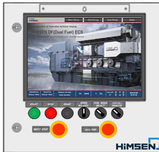
Figure 5.15 Local operating panel
