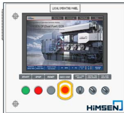
Figure 4-2-4 Local Operating Panel
